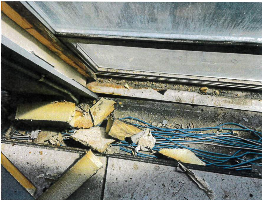
10. Gap at Window Sill
