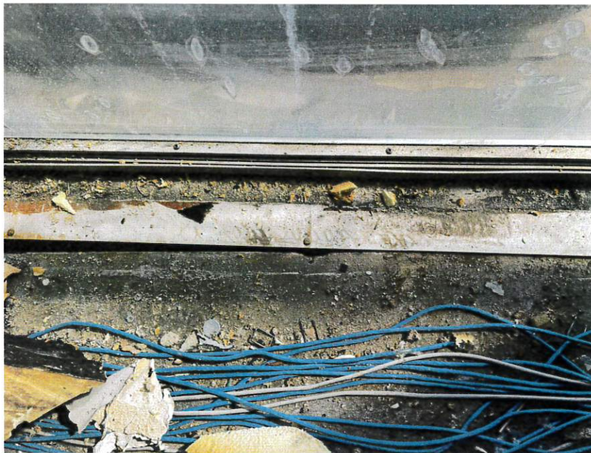
6. Gap at Window Sill
