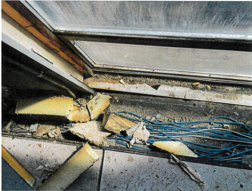
5. Gap at Window Sill
