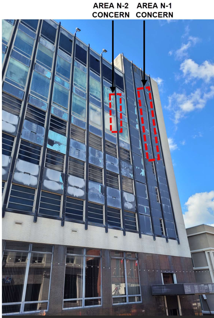
Photo 1: East Wall Elevation Showing Deflecting Wall
